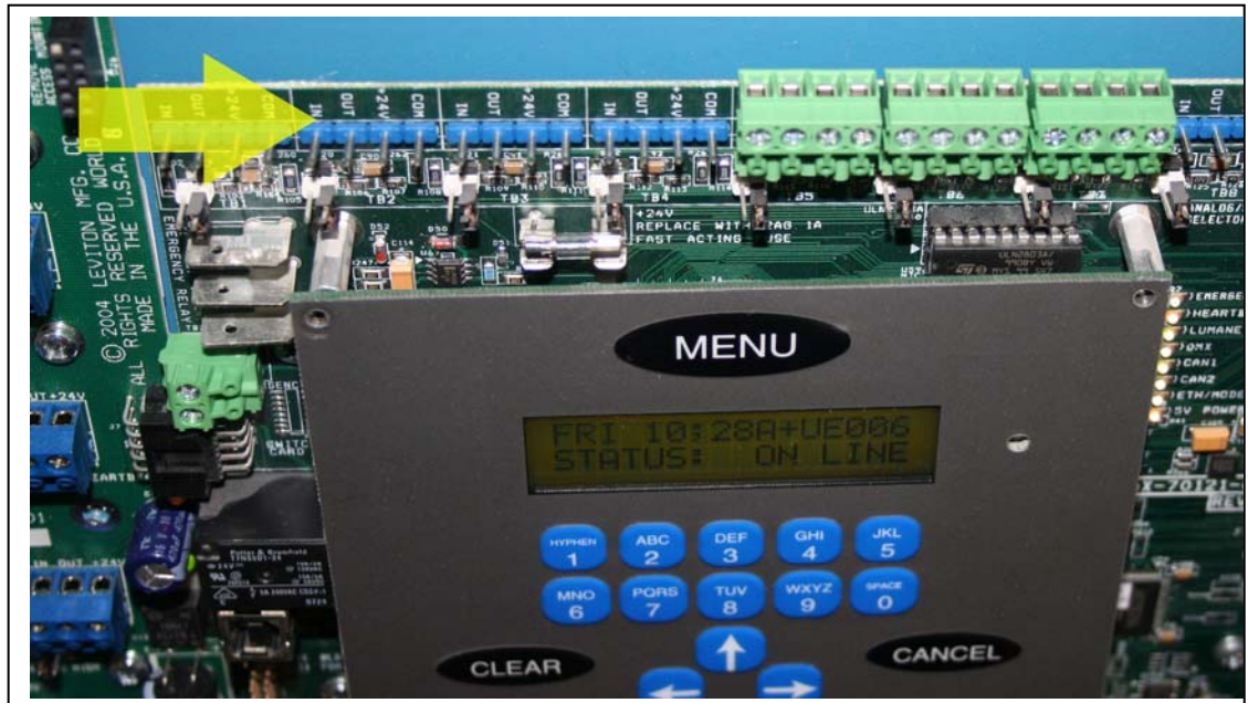
(Image 1-3) 24 and 48 Panels Terminal Block Location – Located Above Control Panel
