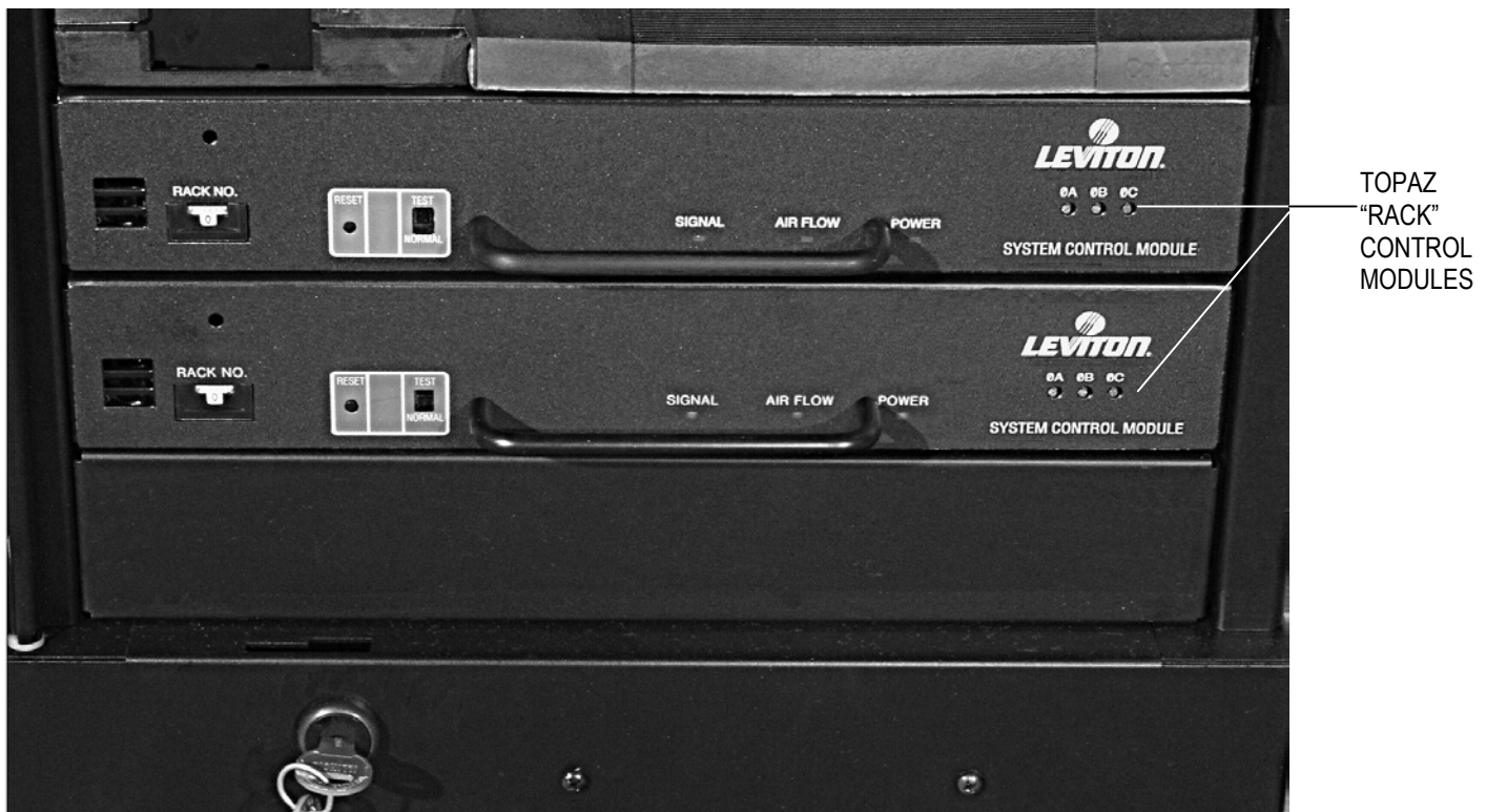
Figure 7 – Control Module Installation
