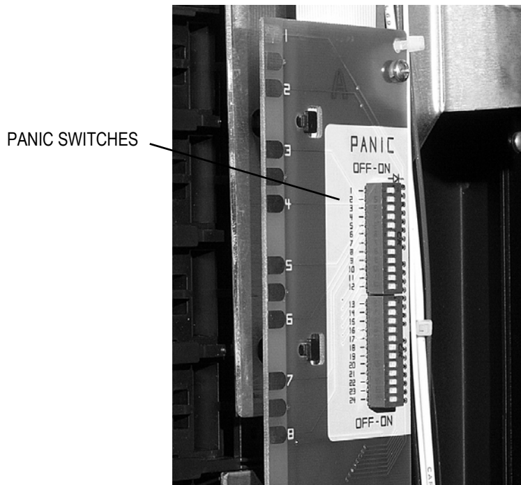
Figure 9 - Panic Switch Location (typical)
