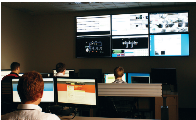
Network operations center (NOC) technicians monitor GigaCenter network performance, power, cooling, and security
