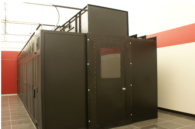
Servers inside a GigaVault, using cold-aisle containment
