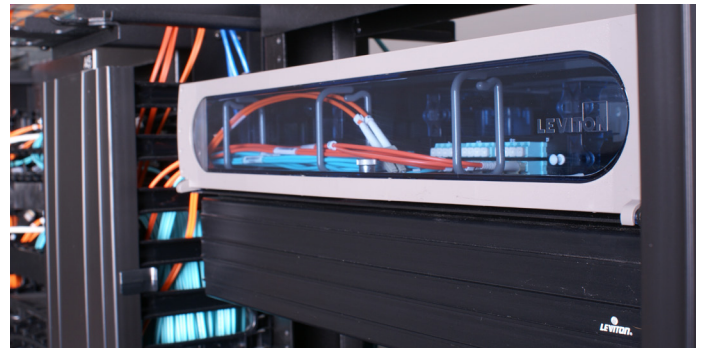
Leviton 2RU Opt-X Ultra Rack-Mount Fiber Enclosure and Versi-Duct Cable Management, in the GigaCenter’s main distribution area
