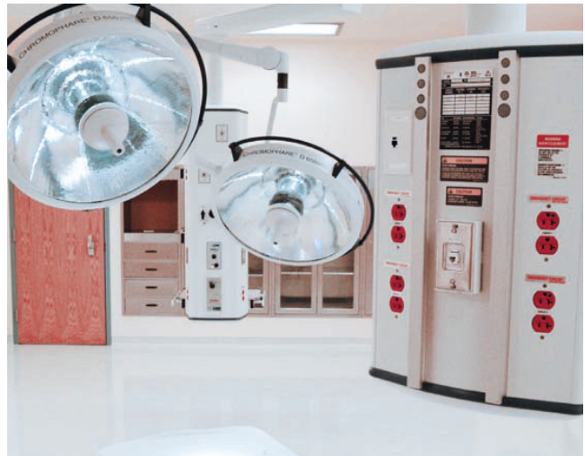
The new OR and cardiac catheterization suites are supported by Leviton copper and fiber systems, ensuring efficient transfer of critical patient data.
