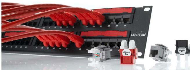
All new data lines are connected with the eXtreme® 6+ CAT 6 UTP system
