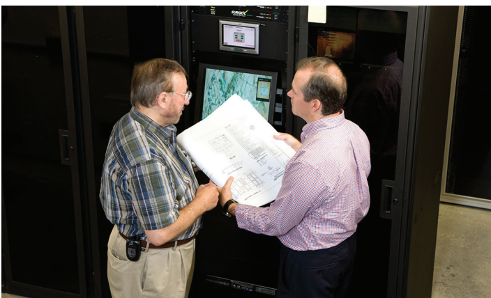
Rich Simmons and Chris Archer review blueprints and terminal data to ensure smooth operations
