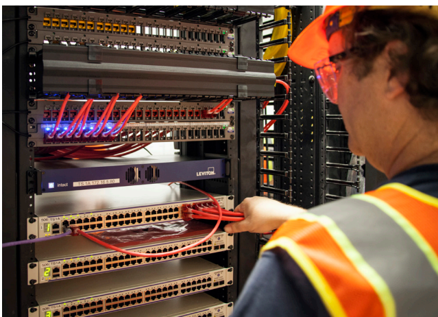
Justin Clausen connecting Intact Secure Cat 6A Copper Patch Cords.
