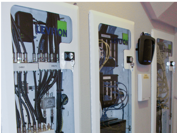
Three Leviton Structured Media® enclosures in the main house
