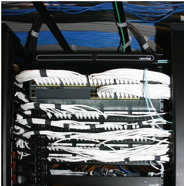
Installed Category 6A FTP Solution.
