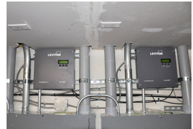
Meters used to monitor resident energy use
