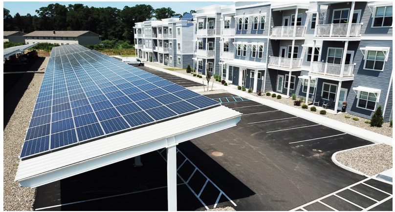
Solar panels on top of the carport help power the community
