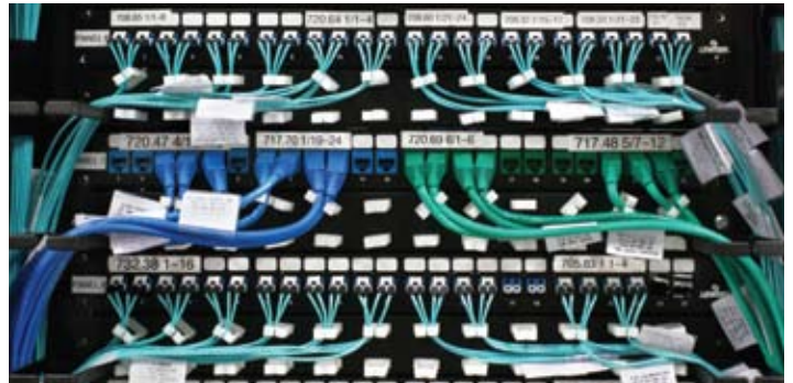
Leviton patch panels, connectors, and patch cords provide copper and fiber connectivity throughout the CBTS data centers
