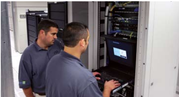
Tony Kidd, senior manager, and Brian Pace, lead technician, manage switches and servers at the Hamilton data center to maintain optimal performance
